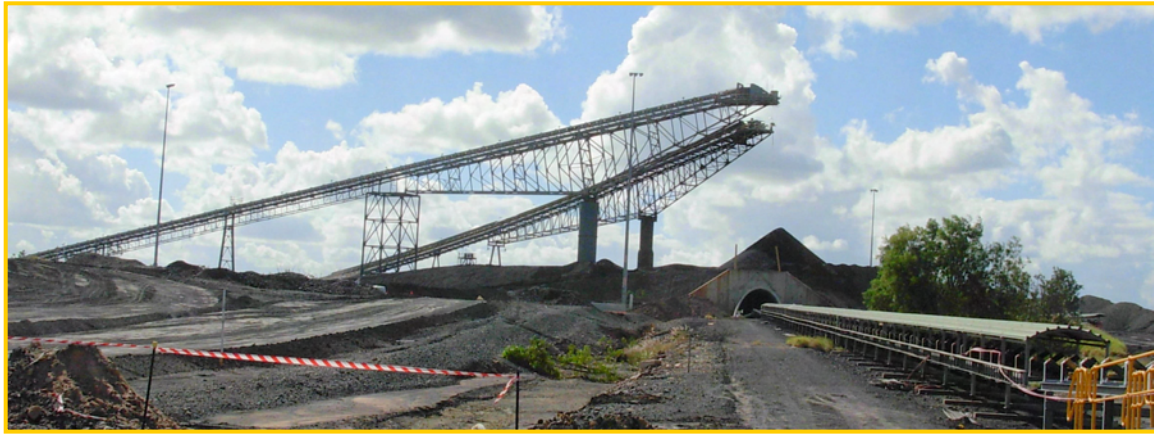
4000 tonnes per hour stockpile conveyor and stockpile reclaim conveyor.
